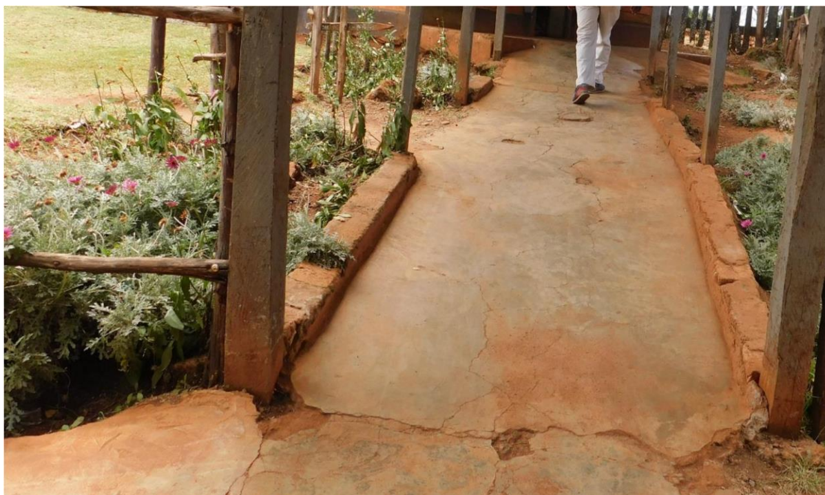
Figure, 4.8 A photograph showing a rough pavement.
